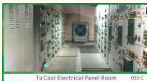
To Cool Electrical Panel Room 055 C
